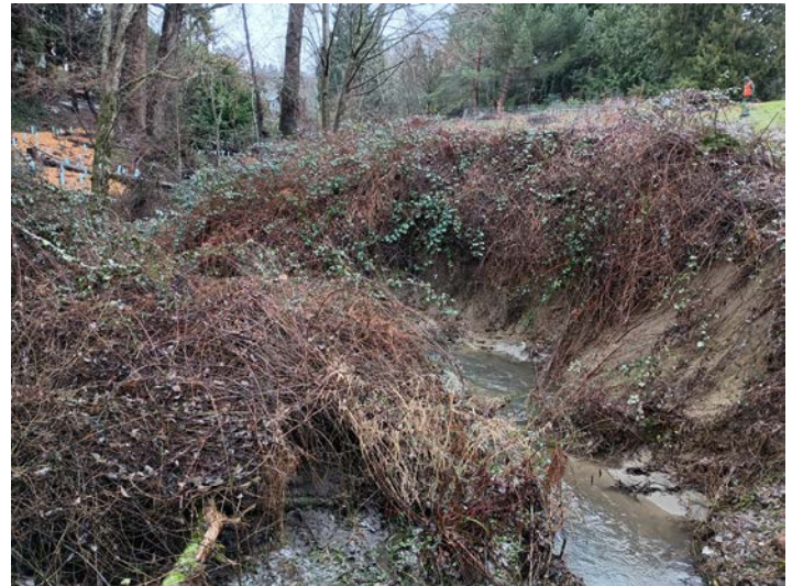
View of Juanita Creek south of Windsor Park; note steep eroding banks and restoration plantings to left
