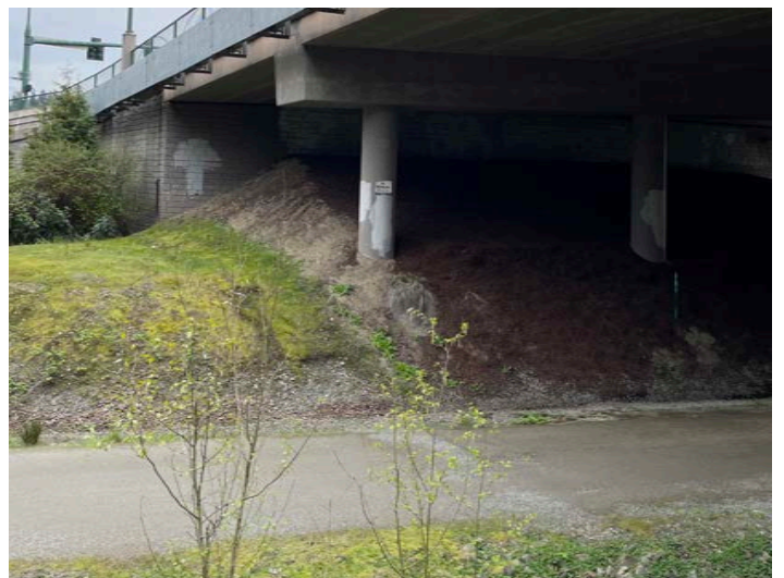
Looking east across the Cross Kirkland Corridor, steep slope and erosion hazard below NE 116th St
