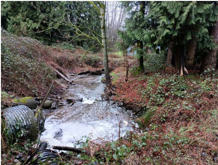
Looking south from NE 145th St at retaining wall supporting I-405, and culvert where Juanita Creek branch emerges
