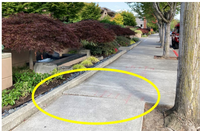
Damaged sidewalk due to tree root uplifting
