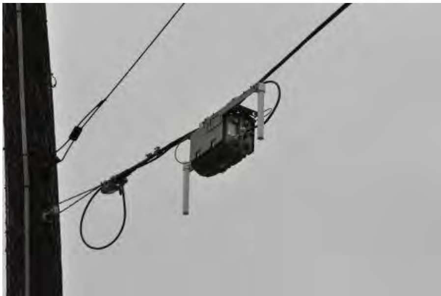
1 Strand Mounted Facility
