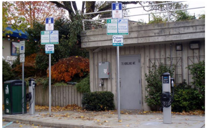
Electric vehicle charging stations at the Marina Parking Lot in downtown Kirkland.
