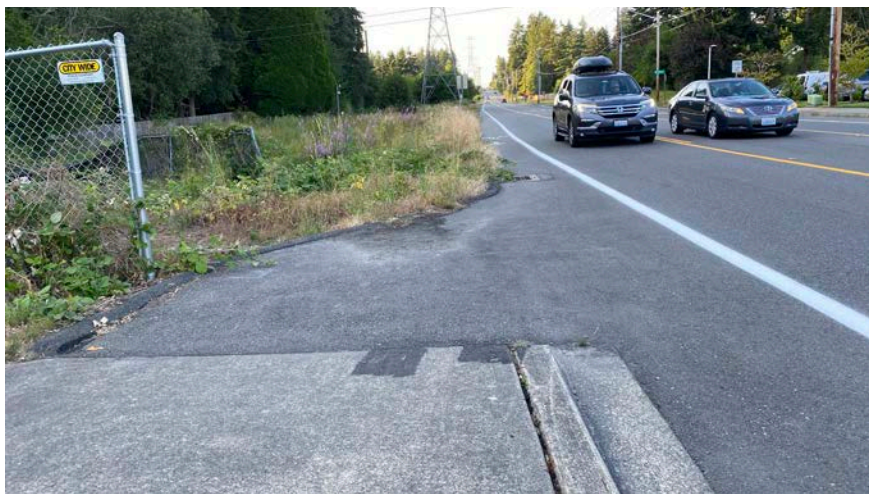
EH04 Sidewalk: 124th Avenue NE from NE 145th Street to city limits
