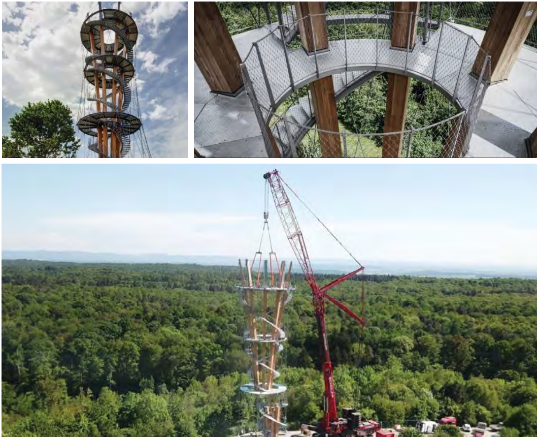
Figure – Pre-assembly of tower on the ground and then lifting complete piece into position
