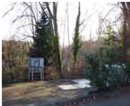
South Bay Lift Station
