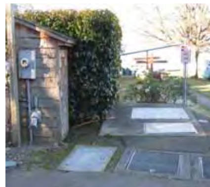
Rose Point Lift Station
