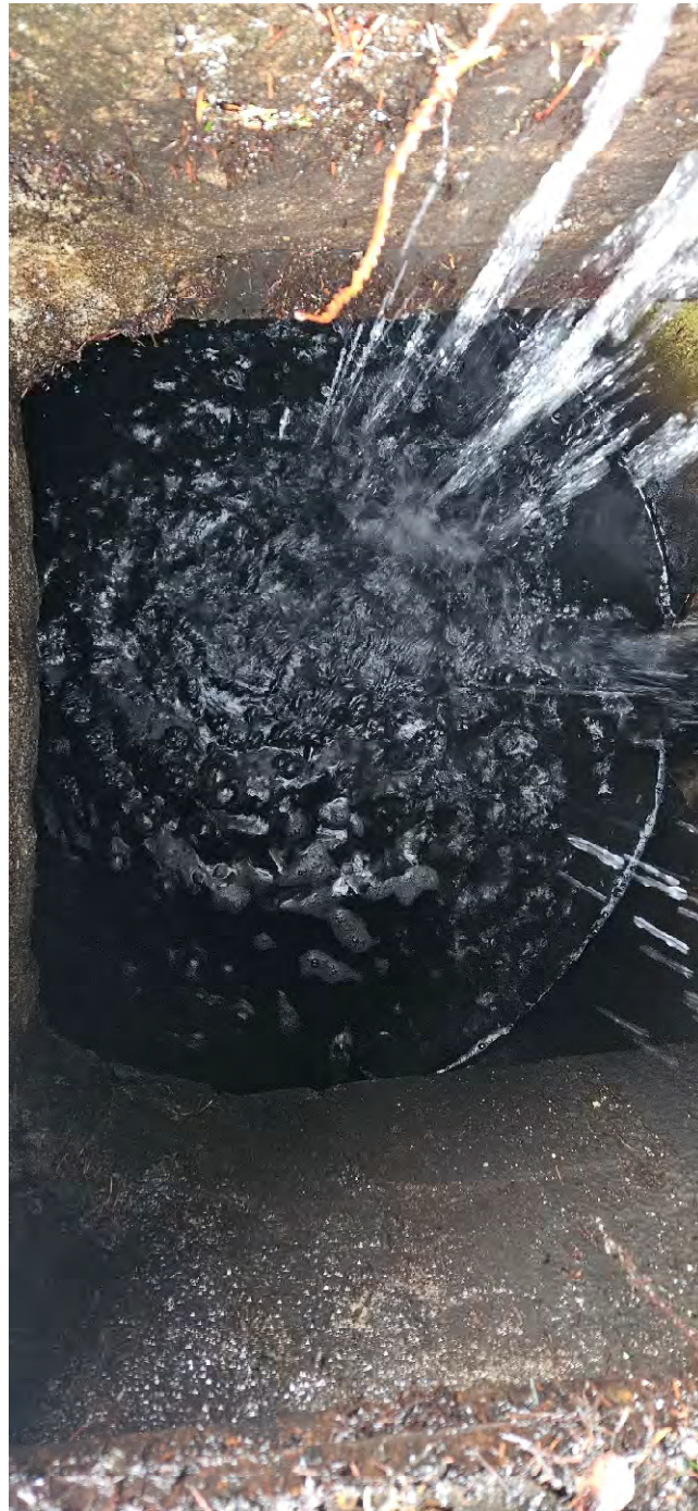
Site 1, CB#10100 –Type 2-48” catch basin
