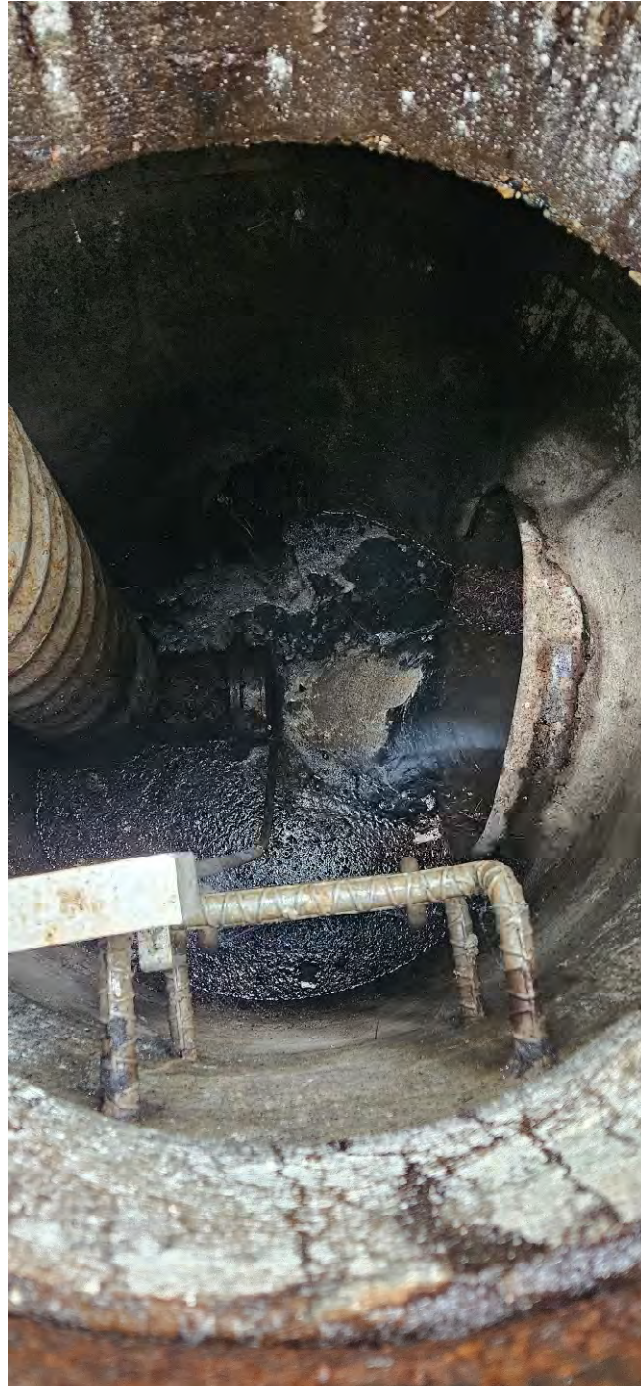
Site 1, CB#9893 – Type 2-48” catch basin in private, backyard area (direction south at top image) flow control riser assembly (left side image), detention tank connector pipe west (right side image)
