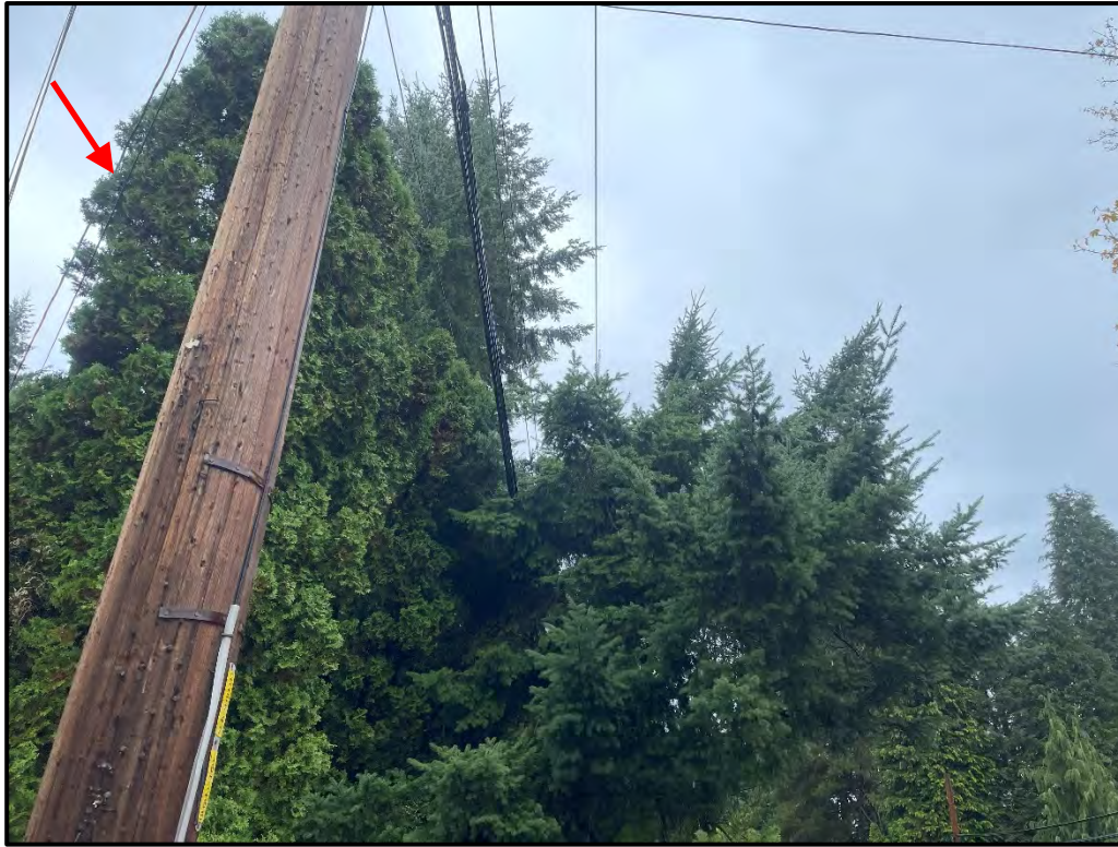
Photograph 3. Overhead utility lines above the trees along 132 nd Ave NE. Tree 216 indicated by the red arrow. Photo taken looking north.
