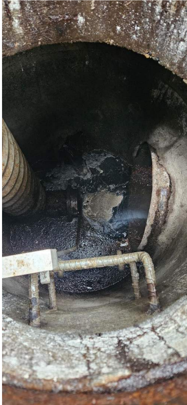
Site 1, CB#9893 – Type 2-48” catch basin in private, backyard area (direction south at top image) flow control riser assembly (left side image), detention tank connector pipe west (right side image)
