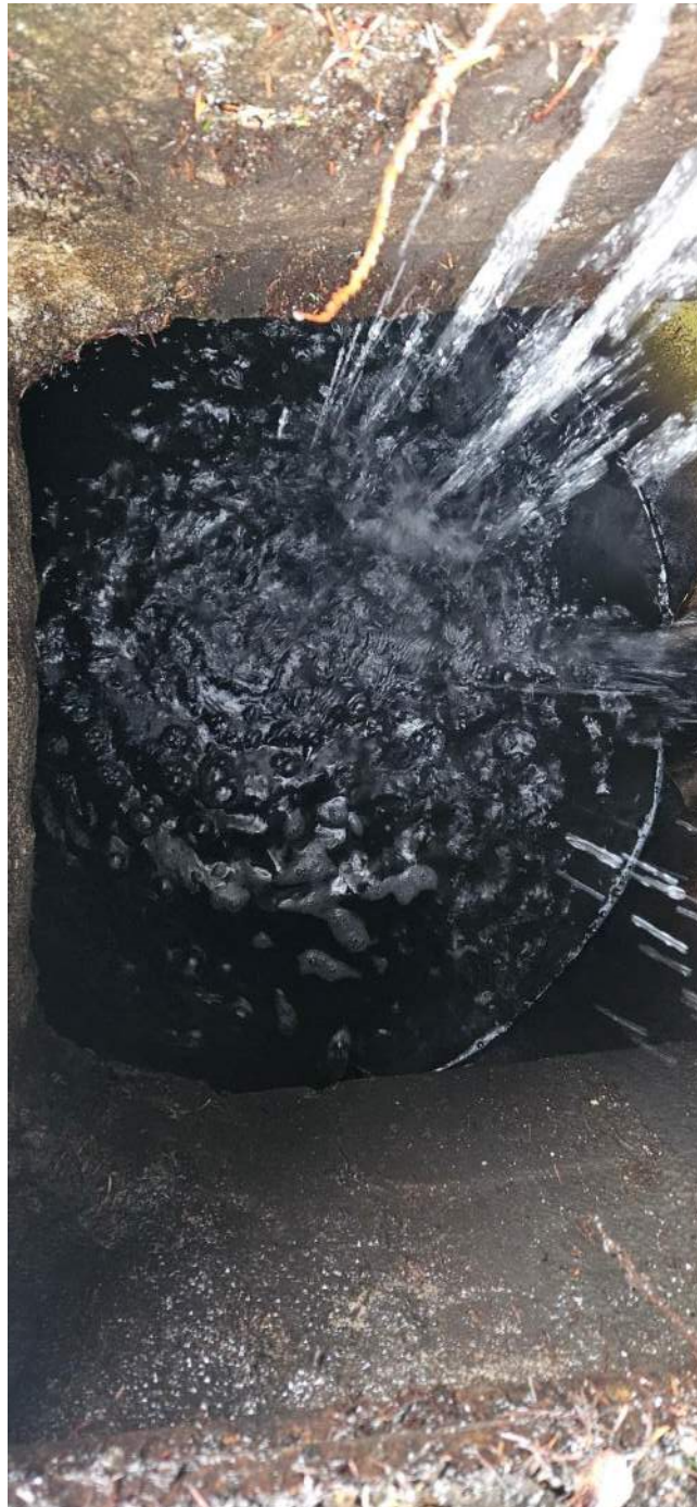
Site 1, CB#10100 –Type 2-48” catch basin
