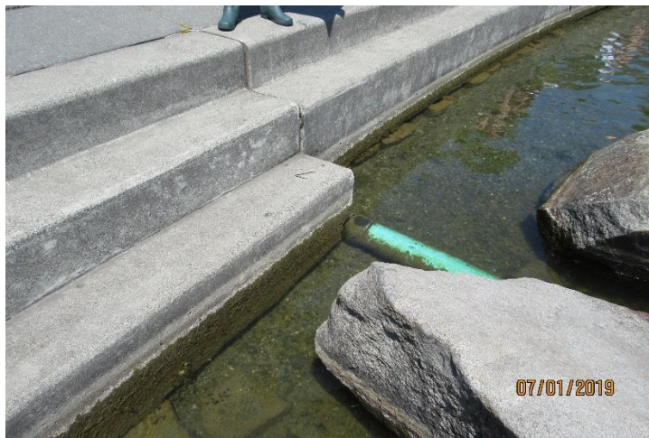
Photo 57. Conc. Steps & Sidewalk (5) Undermining at Toe, Marina Park.
