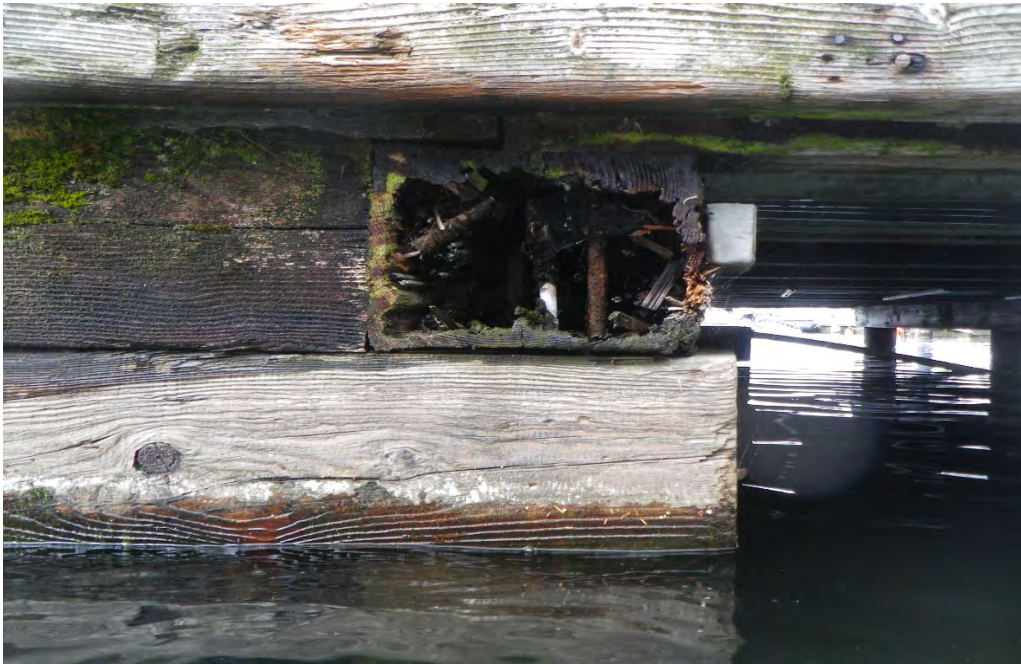
PHOTO No. 7: Bent 3, Row A, Looking West - Note the extensive section loss and visible compression that has resulted from fungal damage of the cap timber.
