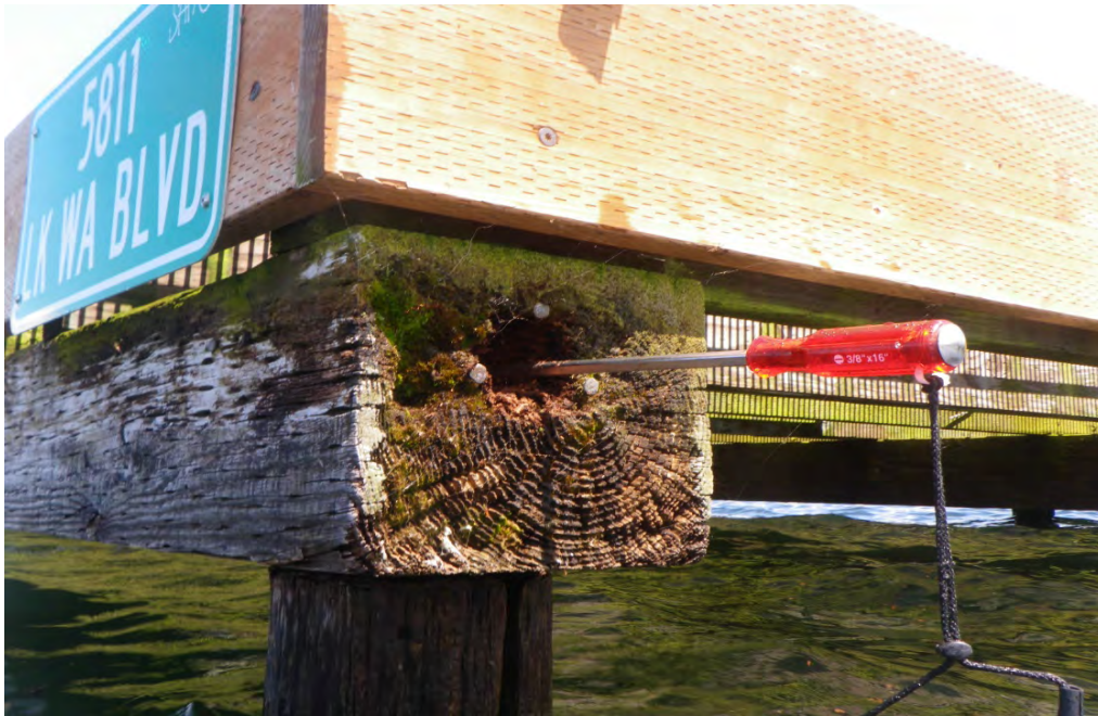
PHOTO No. 7: Bent 33, Row E Pile - Note the screwdriver inserted into a fungal cavity in the end of the pile cap. Inspection estimated a loss of 50% of the member's cross sectional area due to the damage which extends in to the pile top.
