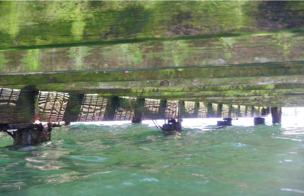
PHOTO No. 9: Bent 32, Looking Southeast - Note the multiple bearing issues at the pile top / cap connections for the substructure piles in this bent. Inspection noted significant deterioration of the tops of these piles. Inspection also noted that shims in several locations are missing or are providing only partial bearing. Also note the generally good condition of the superstructure members with weathering, algae, and water staining.
