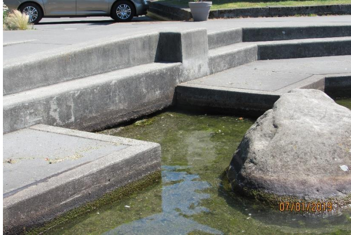
Photo 53. Conc. Steps & Sidewalk (3) Showing Undermining at Toe, Marina Park.
