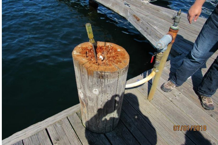
Photo 68. Deteriorated Pile Top on Pier (8), Marina Park.
