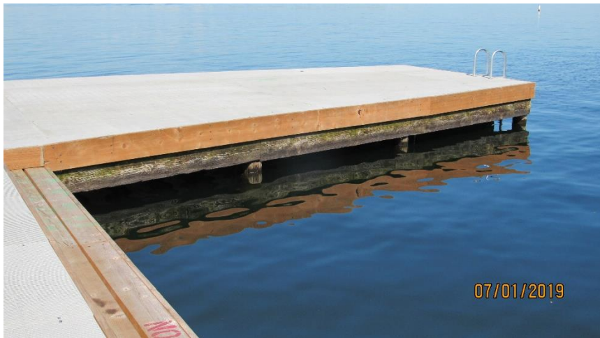
Photo 23. Deteriorated Piles and Pile Caps (8), Houghton Beach Park.
