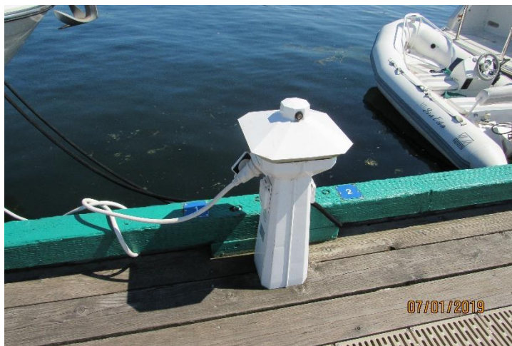
Photo 76. Power Pedestal on Pier (8), Marina Park.
