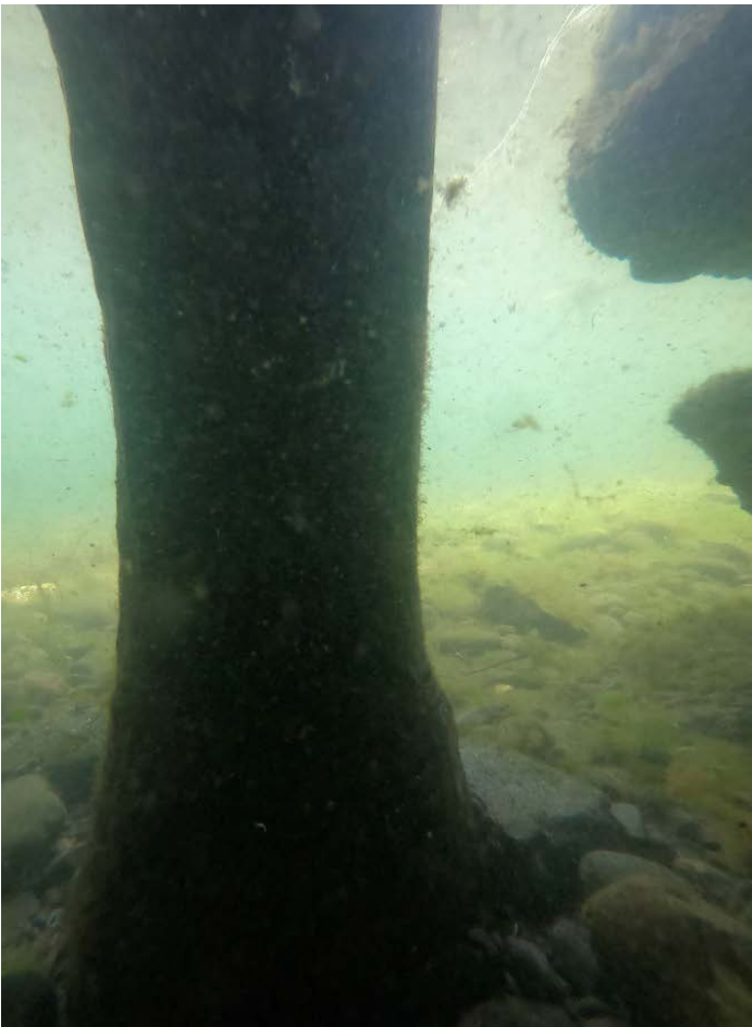
PHOTO No. 8: Bent 37, Row C Pile - Note the thinning of the pile near the mudline, which appears to have been caused by abrasion. Inspection of the timber found it to be generally sound with minor softening of the surface.
