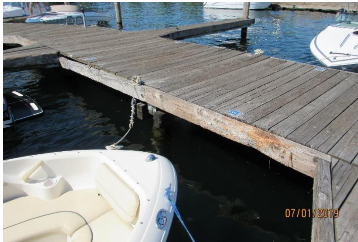
Photo 72. Deteriorated and Damaged Fascia Board and Decking on Pier (8), Marina Park.
