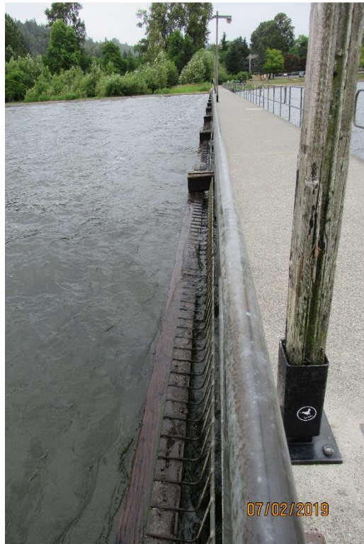
Photo 93. Deteriorated Post of Light Fixture on Pier (1), Juanita Beach Park.
