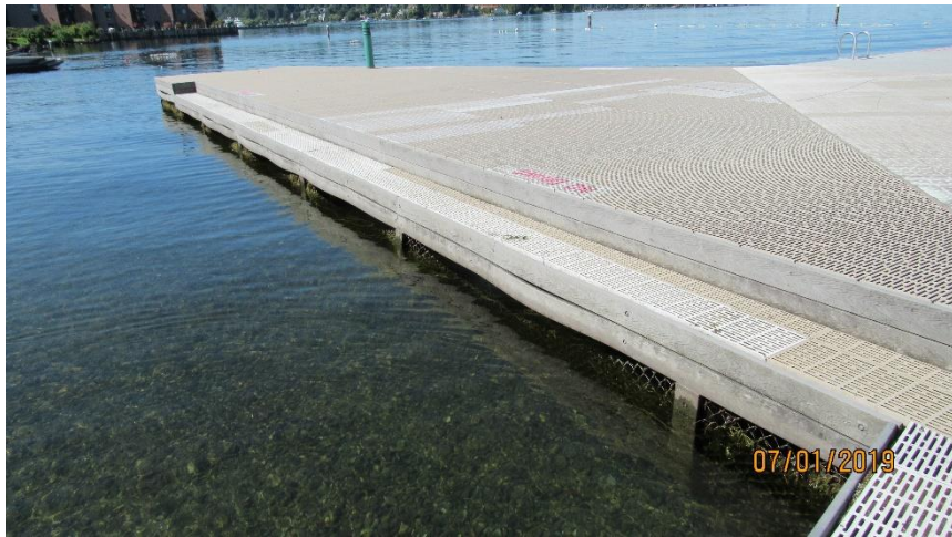
Photo 22. Warped Plastic Timber Fascia on Pier (8), Houghton Beach Park.
