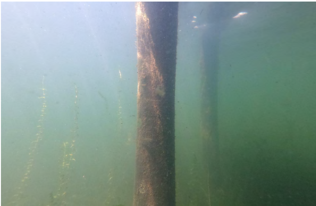
PHOTO No. 7: Bent 10, Row B Pile - Note the overall good condition and light algae growth on the pile in the submerged zone. This was found to be typical of the piles supporting the structure.
