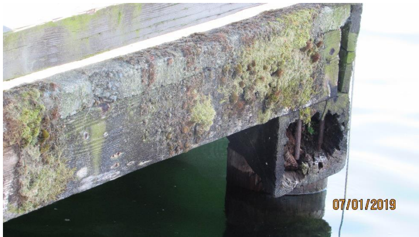
Photo 46. Deteriorated Pile Cap and Fascia Boards on Pier (1), 2 nd Ave. South Dock.
