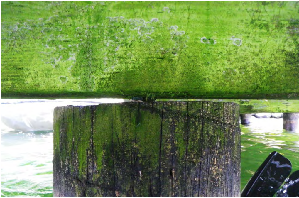
PHOTO No. 5: Bent 8, Row B Pile - Note the gap between the pile top and the cap, as well as the drift pin which is visible. Also note the algae growth on the pile top and cap. Level II cleaning of representative areas found the underlying timber to be in overall good condition with weathering and minor biological degradation.
