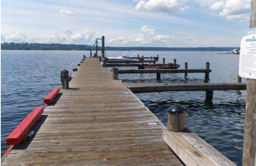
PHOTO No. 5: Western Mooring Finger, Looking Northwest - Note the overall good condition of the timber decking, bull rail, and bench. Also note the piles that extend above the elevation of the deck and the plastic caps covering the pile top end grain on the majority of the piles.
