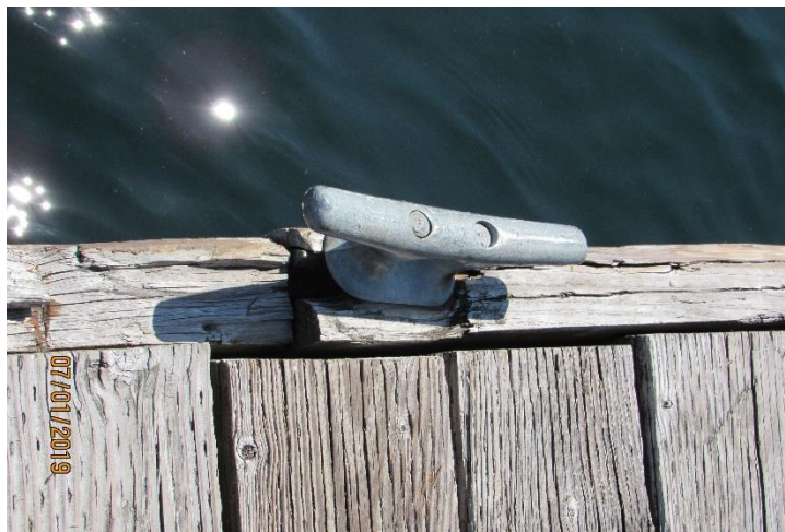
Photo 69. Damaged Fascia Board at a Mooring Cleat Mount Location on Pier (8), Marina Park.
