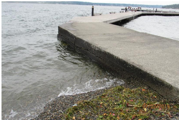
Photo 82. Concrete Pier Cracked (3), Waverly Park.
