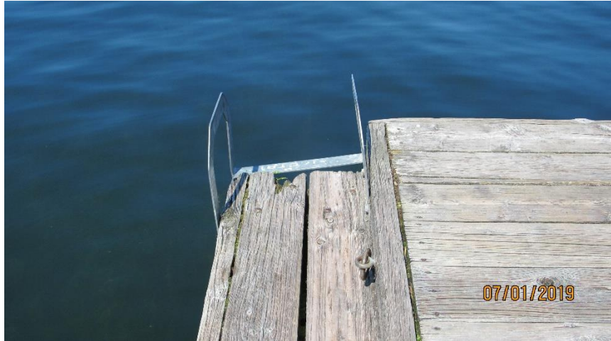
Photo 38. Deteriorated Step Down on Pier (6), Marsh Park.
