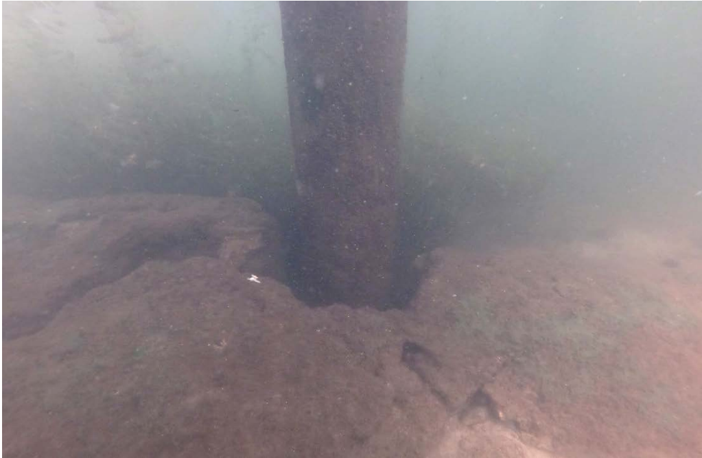
PHOTO No. 9: Bent 46, Row C Pile - Note the generally good condition of the pile, as well as the algae growth covering the surface in the submerged zone. This was found to be typical of the piles throughout the facility in the submerged zone.
