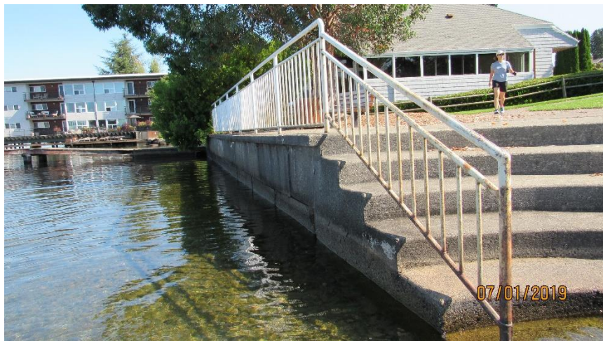
Photo 19. Handrail on Concrete Steps and Sidewalk (8), Houghton Beach Park.
