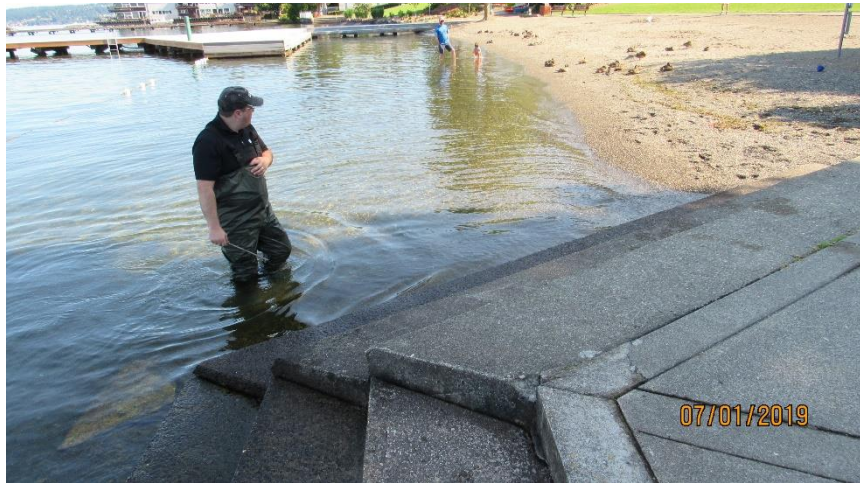
Photo 12. Conc. Crack and Spall damage on Conc. Steps (6), Houghton Beach Park.
