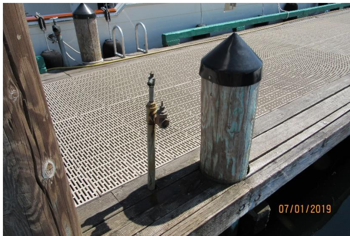
Photo 75. Hose Bib for Potable Water without Handles on Pier (8), Marina Park.
