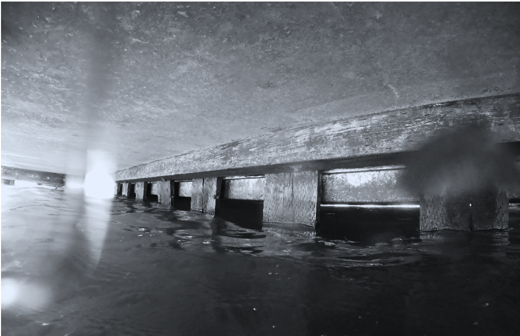
PHOTO No. 13: Bent 40 - 42, Row B, Looking West - Note the step-down in the concrete deck at the intersection of the water-walk and the swim platform along Row B. Also note the vertical boards, assumed to be a wave screen, which are secured to the underside of the deck. Investigation noted that a number of the boards appear to have gone missing or to have been removed.
