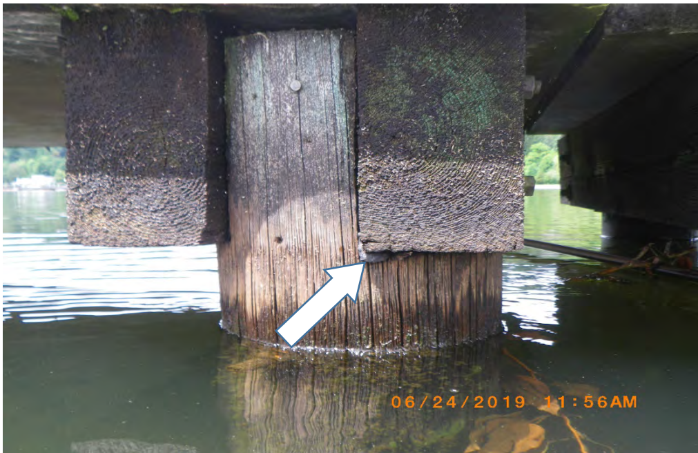
PHOTO No. 3: Bent 9, Row A, Pile / Cap Connection - Note the construction notches on both sides of the pile to provide a seat for the cap timbers. Also note the apparent field treatment of the pile at the notched areas (Refer to arrow). Inspection found that typically the piles have sustained weathering and/or minor biological degradation from the top down to low water.
