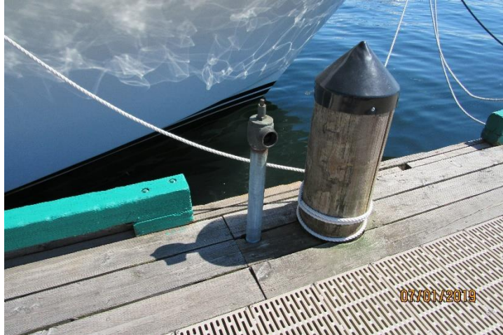
Photo 74. Fire Standpipe Missing Caps and Handles on Pier (8), Marina Park.
