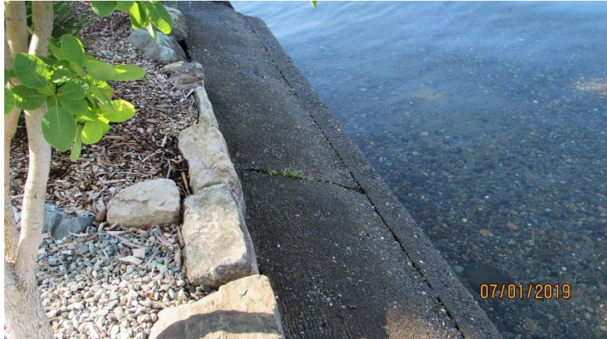
Photo 16. Cracked Concrete Revetment (8), Houghton Beach Park.
