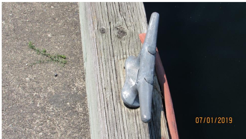
Photo 46. A Loose Cleat on Pier (1), 2 nd Ave. South Dock.
