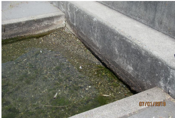
Photo 54. Conc. Steps & Sidewalk (3) Showing Undermining at Toe, Marina Park.
