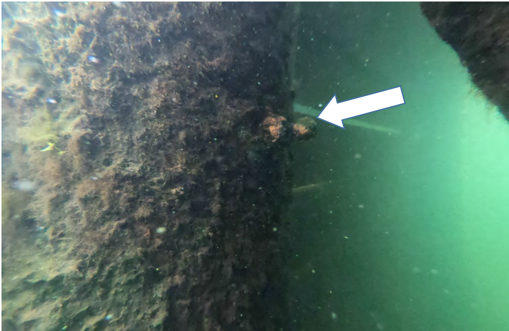
PHOTO No. 13: Bent 18, Row A Pile - Note the moderate corrosion evident on the surface of this thru-bolt that secures a diagonal wavebreak. Also note the typical algae growth and the typical good condition of pile in submerged zone.
