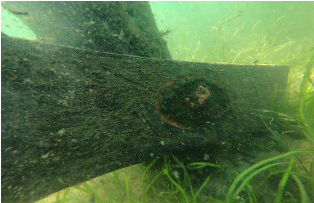
PHOTO No. 5: Bent 15, Row A Pile - Note the 3x10 treated diagonal brace timber attached to the pile at the mudline. Inspection found the brace timbers to be in generally good condition with minor biological degradation of the timber surface and minor to moderate corrosion on the attachment hardware.
