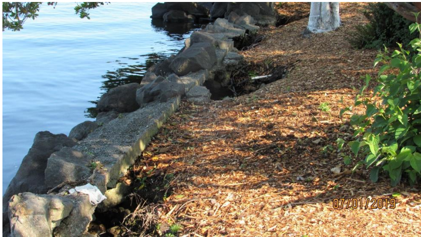
Photo 5. Voids behind Riprap (3), Houghton Beach Park.
