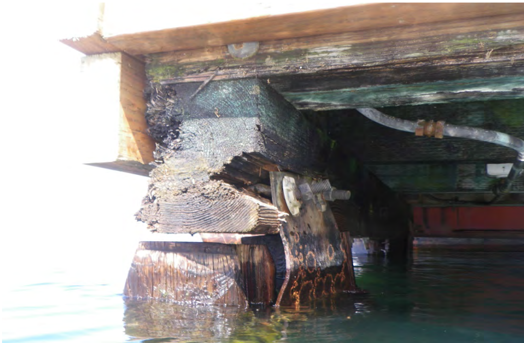
PHOTO No. 17: Bent 35, Row B Pile - Inspection noted this mechanical damage to the end of the cap which has been estimated at 25% loss. The structure has apparently sustained impact damage resulting in damage to the steel bracket securing the batter pile, as well as exposing the attachment bolts.
