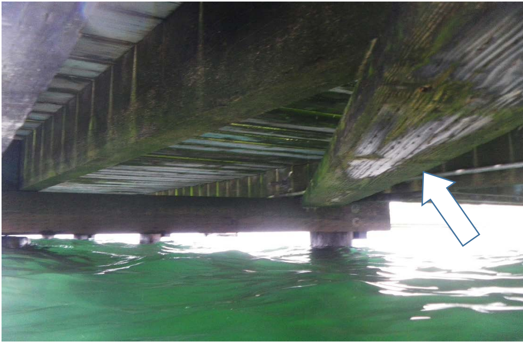
PHOTO No. 21: Bent 82 to Bent 83, Superstructure - Note the diagonal brace located at the elevation of the cap (refer to arrow) and extending diagonally from the Row A Pile to the Row B Pile. Also note the overall good condition of the cap, stringers, and the under-surface of the deck timber.
