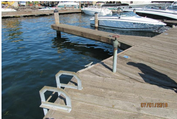
Photo 73. Safety Ladder, Cleat, and Fire Standpipe on Pier (8), Marina Park.
