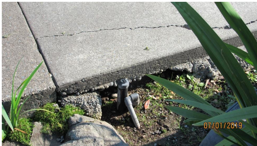
Photo 8. Cracked and Undermined Sidewalk (4), Houghton Beach Park.
