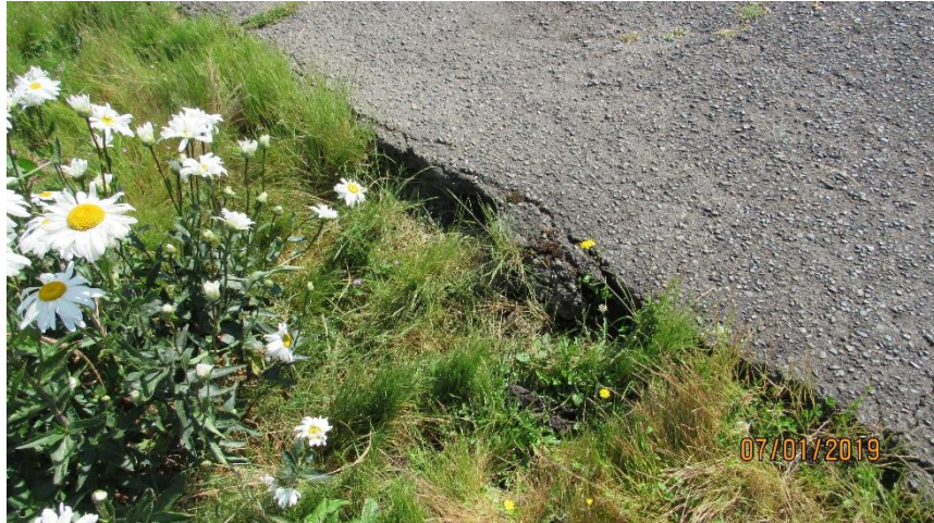
Photo 27. Evidence of Erosion on Riprap Bank & Asphalt Pathway (2), Marsh Park.
