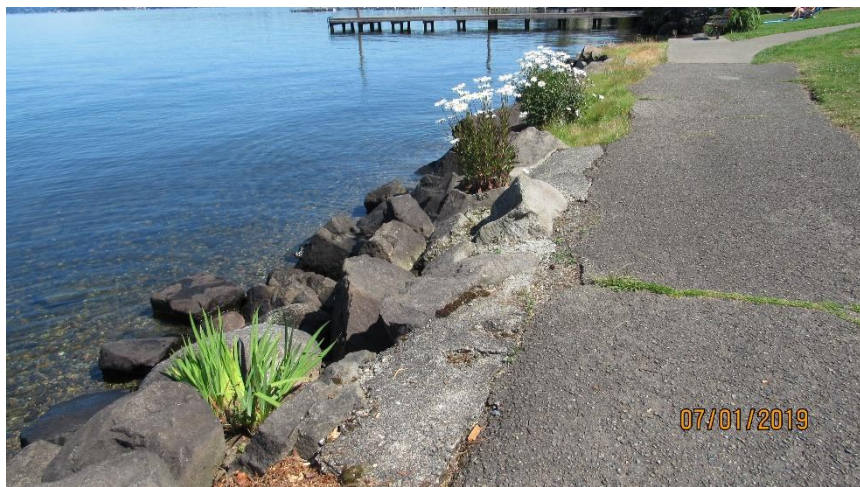
Photo 26. Riprap Bank & Asphalt Pathway (2) Looking North, Marsh Park.
