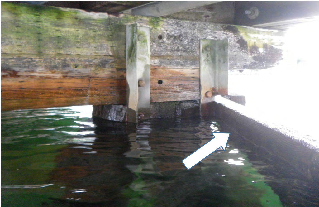
PHOTO No. 9: Bent 38, Row A Vertical and Batter Pile - Note the galvanized angle brackets used to connect the batter pile top (left), and the vertical pile top (right) to the glu-lam cap. Also note the diagonal wavebreak which is attached to the vertical pile (refer to arrow) and the algae and water staining on the glu-lam cap.
