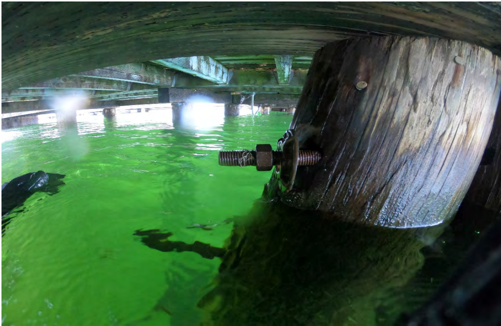
PHOTO No. 9: Bent 18, Row A Batter Pile - Inspection noted this loose hardware securing the batter pile to the vertical pile. Several loose batter pile connections were identified throughout the structure. Additionally, no blocking was found on any of the batter piles throughout the pier, between the top of the piles and the superstructure.
