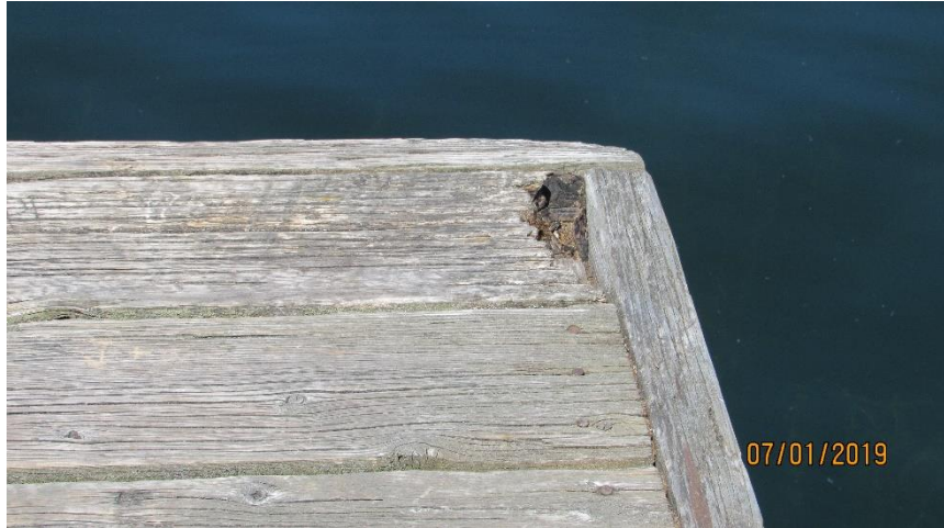
Photo 40. Deteriorated Decking and Fascia Board on Pier (6), Marsh Park.
