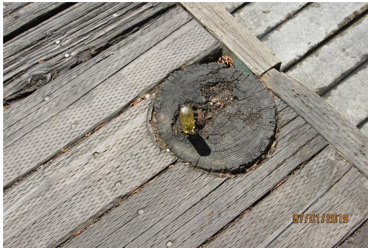
Photo 63. Deteriorated Pile Top on Boat Ramp Pier (7), Marina Park.
