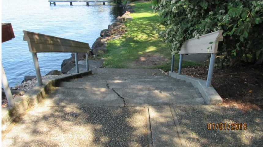
Photo 33. Cracked Concrete Steps (4), Marsh Park.
