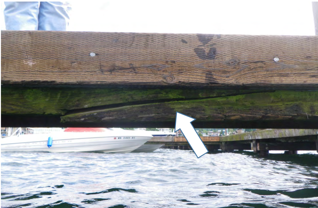
PHOTO No. 19: Bent 88, Row B-C, North Perimeter Stringer - Note the failure of this perimeter stringer, which is one of two stringers providing support for the deck. Inspection also noted the newer members sistered to and secured to the damaged stringer.
