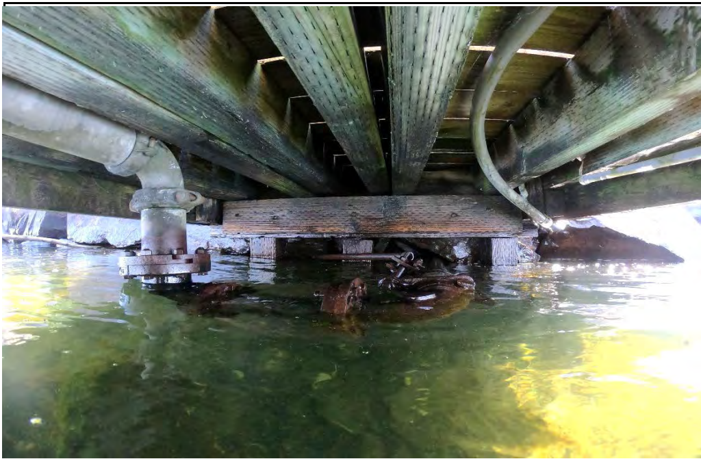
PHOTO No. 3: Bent 1, Looking East - Note the three 6x6 posts supporting Bent 1 and the overall good condition of the superstructure members. Inspection of the posts found them to be in generally good condition but noted that all three are bearing directly on large rock. Additionally, the center, Row B post, was found to be non-bearing beneath the cap.
