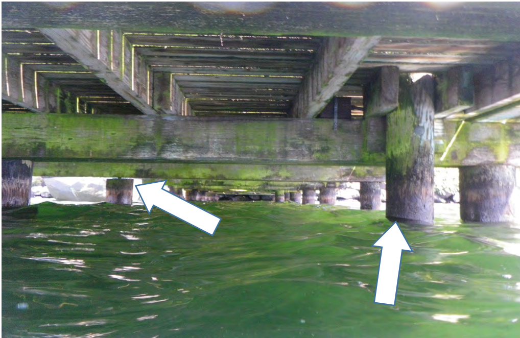
PHOTO No. 3: Bent 10, Looking East- Note the overall good condition of the piles and superstructure members, with minor water staining and algae growth. Also note the right arrow indicating the Bent 9.1 light post and the left arrow indicating the non-bearing condition of the Bent 8, Row B pile.
