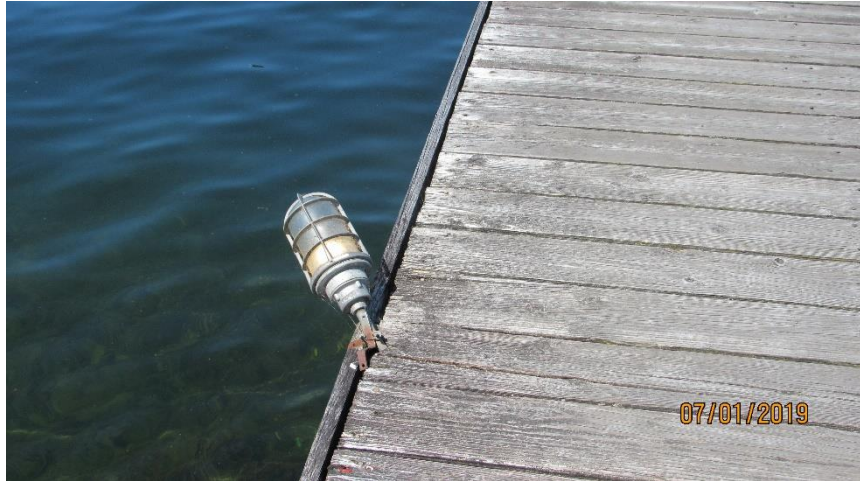
Photo 43. Damaged Light Fixture on Pier (6), Settlers Landing.
