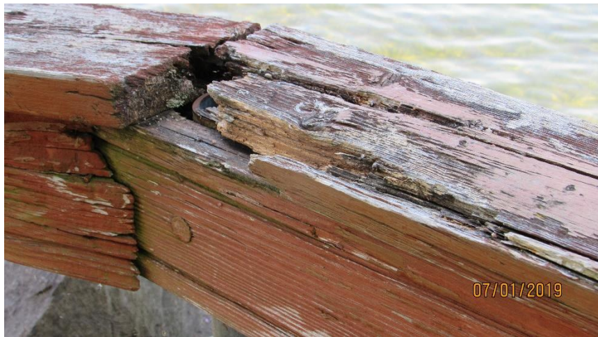
Photo 32. Deteriorated Handrail (4), Marsh Park.
