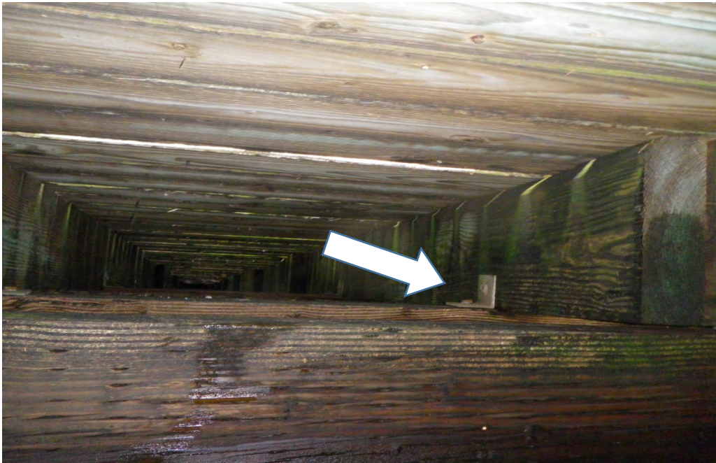
PHOTO No. 3: Bent 17 Superstructure - Note the overall good condition of the pile cap, stringers, and the underside of the decking within the pier. Also note the good condition of the galvanized angle bracket securing the stringer to the cap.
