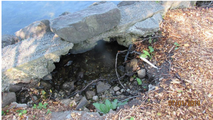
Photo 6. A Large Void behind Riprap (3), Houghton Beach Park.
