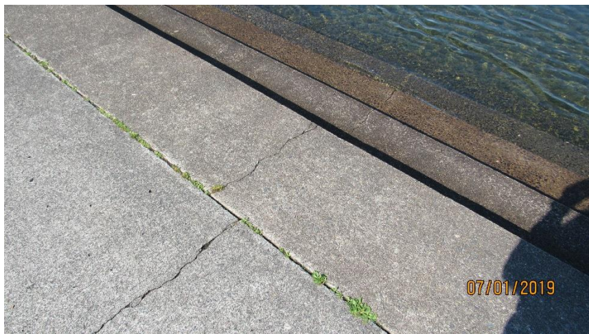
Photo 9. Cracked Steps (4), Houghton Beach Park.
