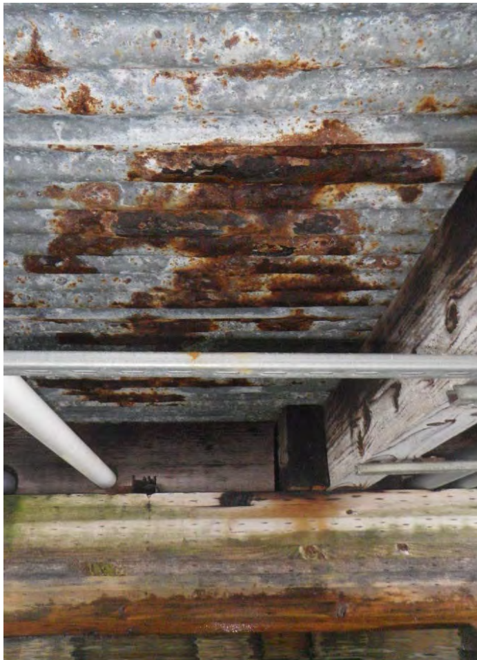
PHOTO No. 6: Bents 39-40, Corrugated Deck Pan - Note the corrosion of the galvanized sub pan at this location. Overall, the condition of the sub-pan was found to be generally fair with an estimated 20- 25% of the surface found to have localized surface corrosion with areas of perforation.
