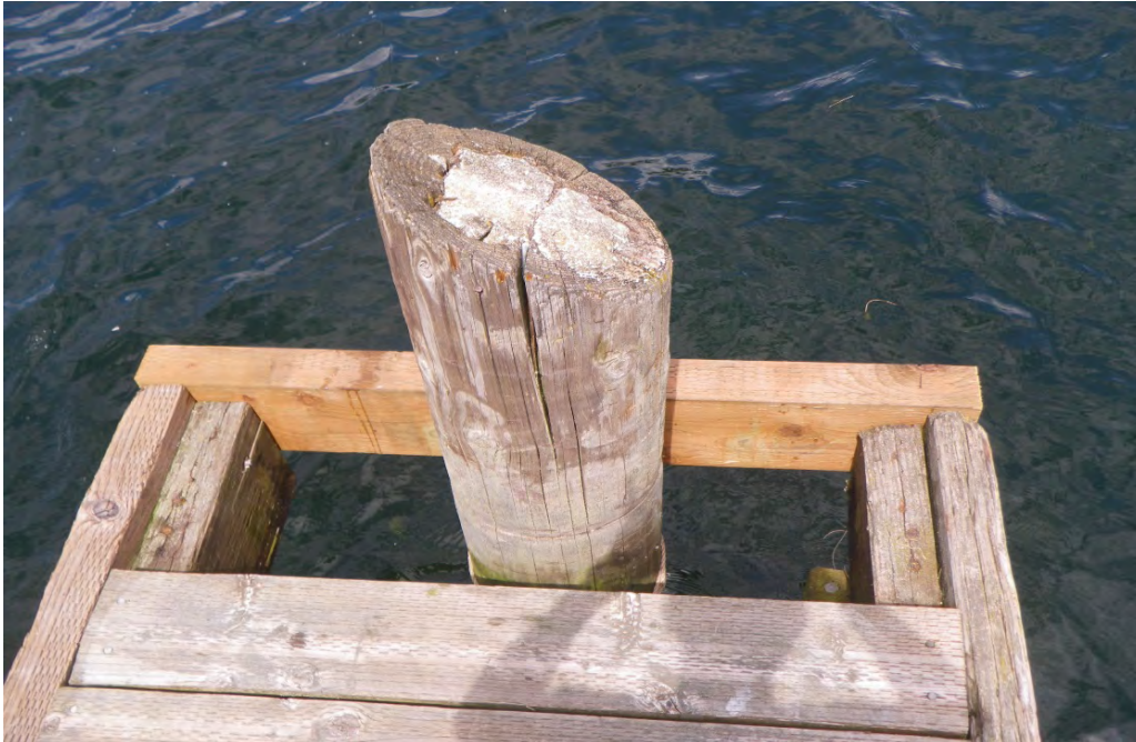
PHOTO No. 7: Bent 88, Row E Pile - Note the center of the pile has been filled with concrete grout. Inspection of the pile estimated that the pile has internal fungal damage below the concrete which extends down several feet. Also note the missing plastic cap and the new edge member indicating on-going maintenance of the framing and decking at this location.
