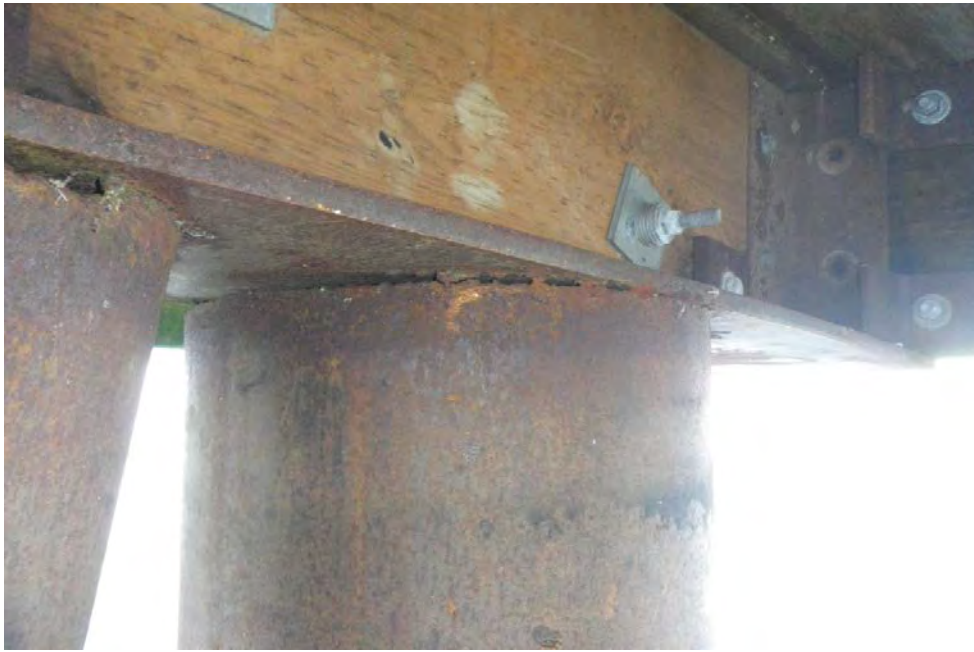
PHOTO No. 13: Bent 88, Row D, Steel Sleeved Pile - Note the minimal amount of tack welds securing the top of this steel pipe pile sleeve to the steel plate on the connection bracket. Also note the minor surface corrosion of the uncoated steel above water.
