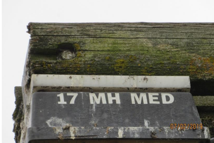
Photo 93. Deteriorated Light Fixture on Pier (1), Juanita Beach Park.
