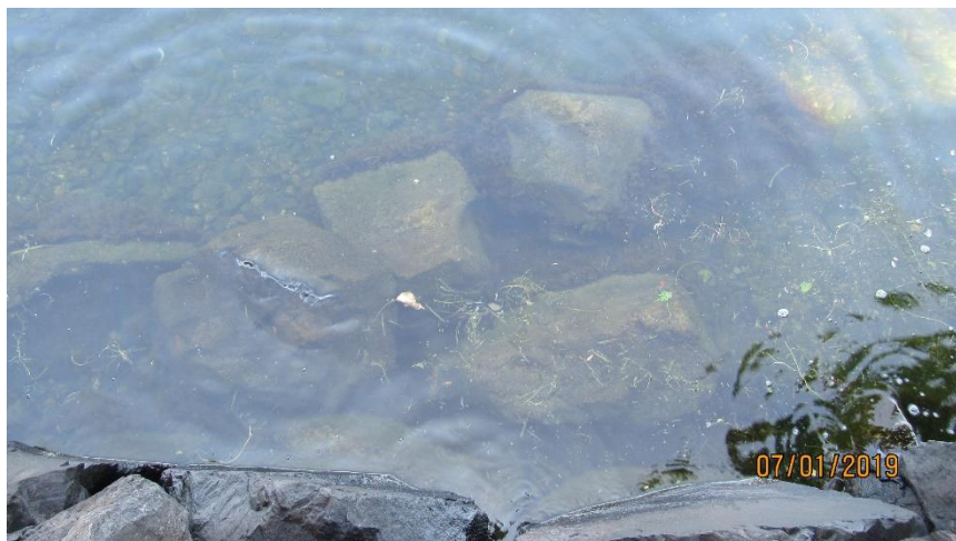
Photo 35. Displaced Rocks from Riprap Bulkhead (5), Marsh Park.
