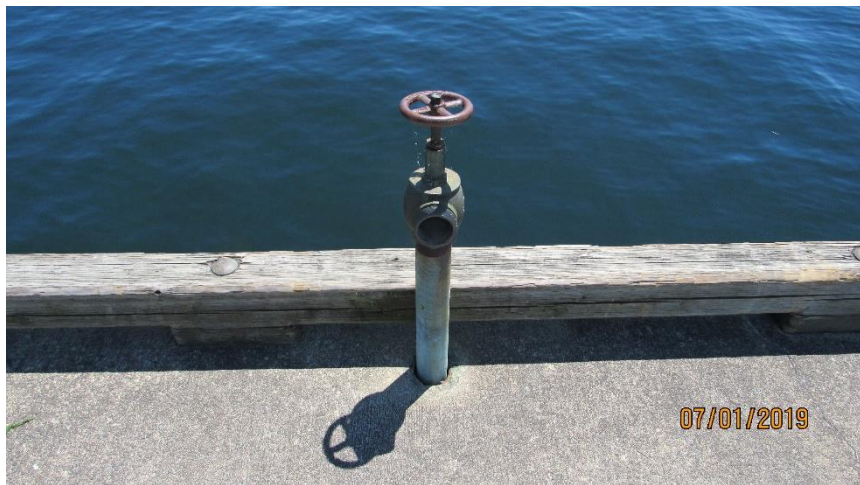
Photo 48. Fire Standpipe on Pier (1), 2 nd Ave. South Dock.
