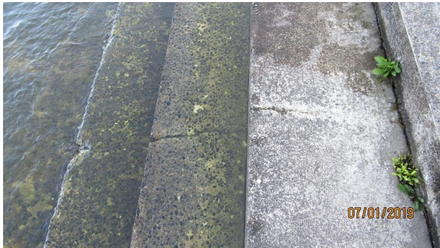
Photo 11. Conc. Crack and Spall damage on Curved Conc. Steps (5), Houghton Beach Park.
