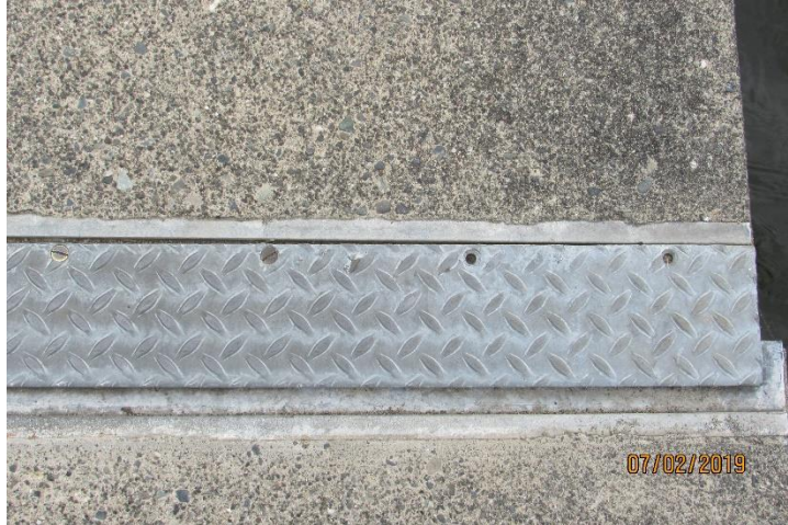
Photo 91. Missing Screws on a Steel Plate at an Expansion Joint on Pier (1), Juanita Beach Park.
