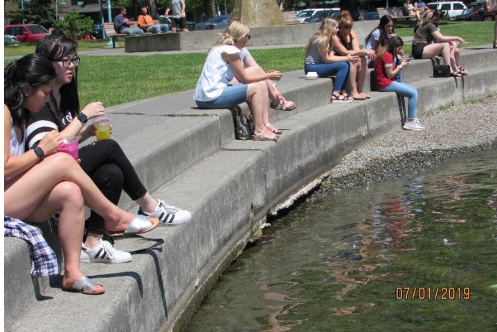
Photo 56. Conc. Steps & Sidewalk (5) Undermining at Toe, Marina Park.
