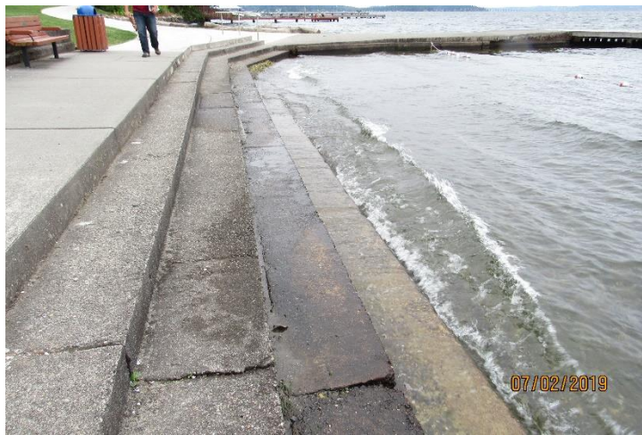
Photo 83. Concrete Steps & Sidewalk Cracked (4), Waverly Park.
