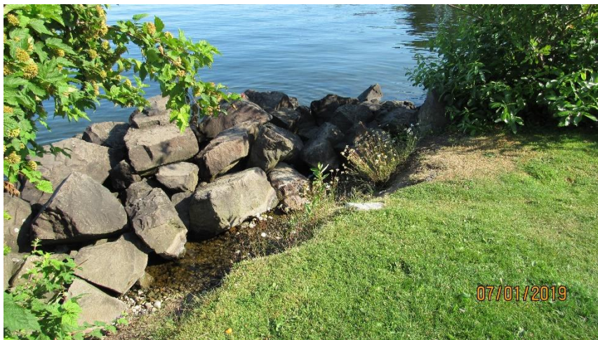
Photo 2. Riprap Bank Slope (1) Slightly Eroded, Houghton Beach Park.
