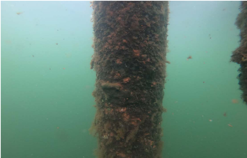
PHOTO No. 11: Bent 88, Row D, Steel Sleeved Pile - Note the algae growth, surface corrosion and rust nodules visible on the steel pipe pile sleeve which appears to have been installed over the top of the original timber pile. No apparent lag bolts or other hardware was noted securing this sleeve to the timber stub.
