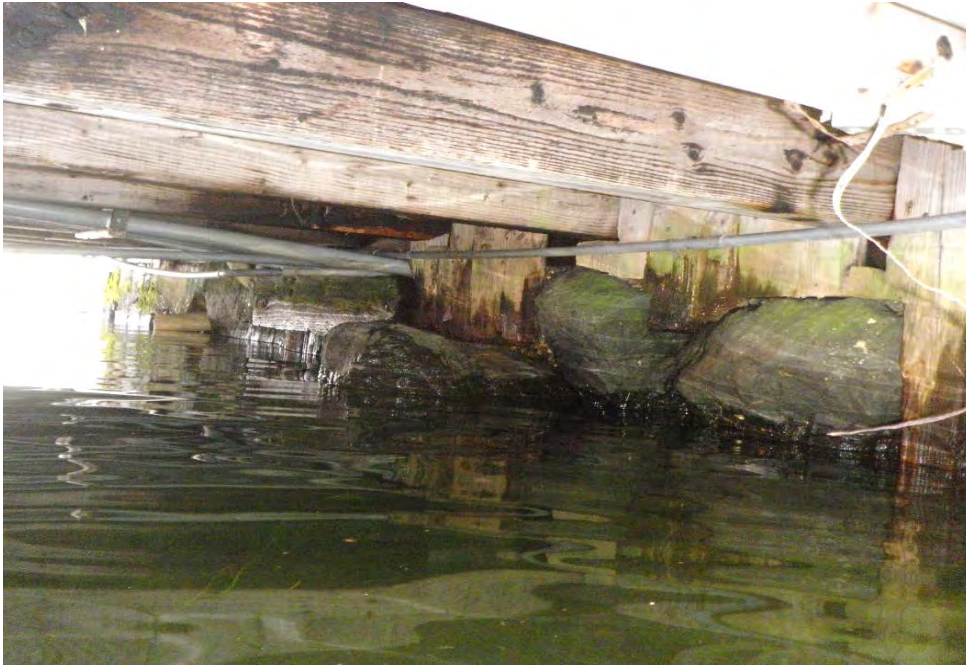
PHOTO No. 5: Shore Abutment, Looking North - Note the deterioration of the vertical lagging timbers used as a backwall to contain the shoreward soils. Inspection did not identify any apparent loss of back fill.
