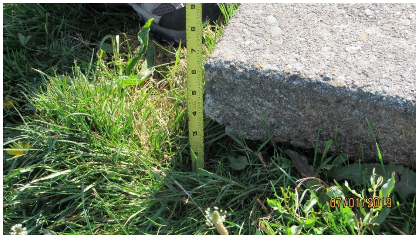
Photo 28. A Void below Concrete Bench Foundation (2), Marsh Park.
