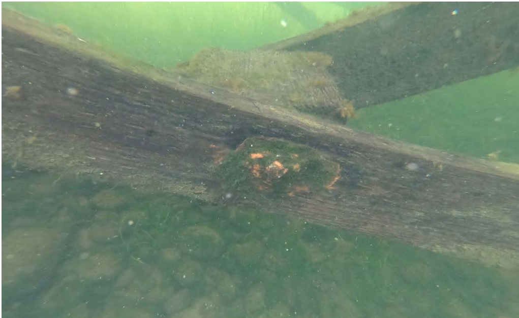
PHOTO No. 9: Bent 4 -5, Row A, Diagonal Bracing, Looking South - Note the moderate corrosion of the thru-bolt and the use of a center block at the mid-connection on this set of diagonal braces. Inspection found the bracing timbers to be in generally good condition with no evidence of any gross damage.
