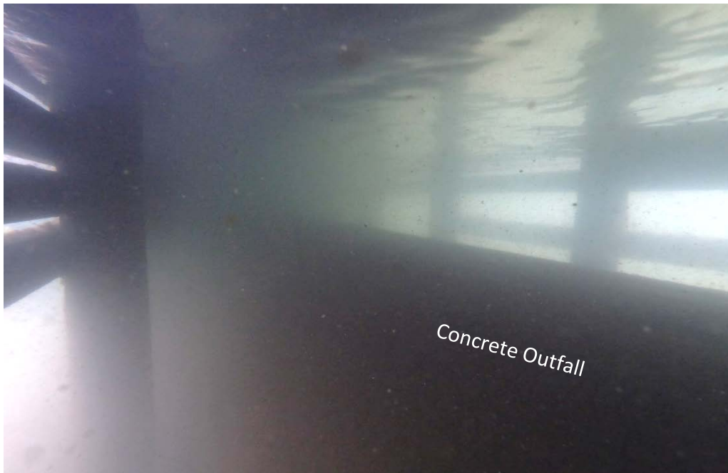
PHOTO No. 5: Bent 16, Looking East - Note the large concrete storm sewer outfall which runs the length of the structure. Also note the fender system running along the north and south perimeter of the pier. The presence of the outfall resulted in limited access to the piles and superstructure members.
