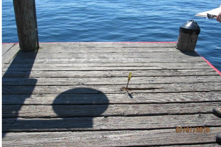
Photo 62. Deteriorated Decking on Boat Ramp Pier (7), Marina Park.
