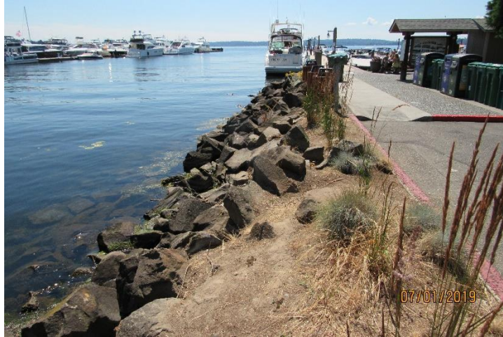
Photo 50. Riprap Bank Slope (1) Looking Southwest, Marina Park.
