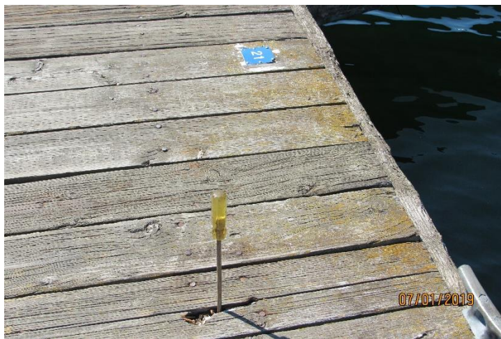
Photo 70. Deteriorated and Damaged Fascia Board and Decking on Pier (8), Marina Park.
