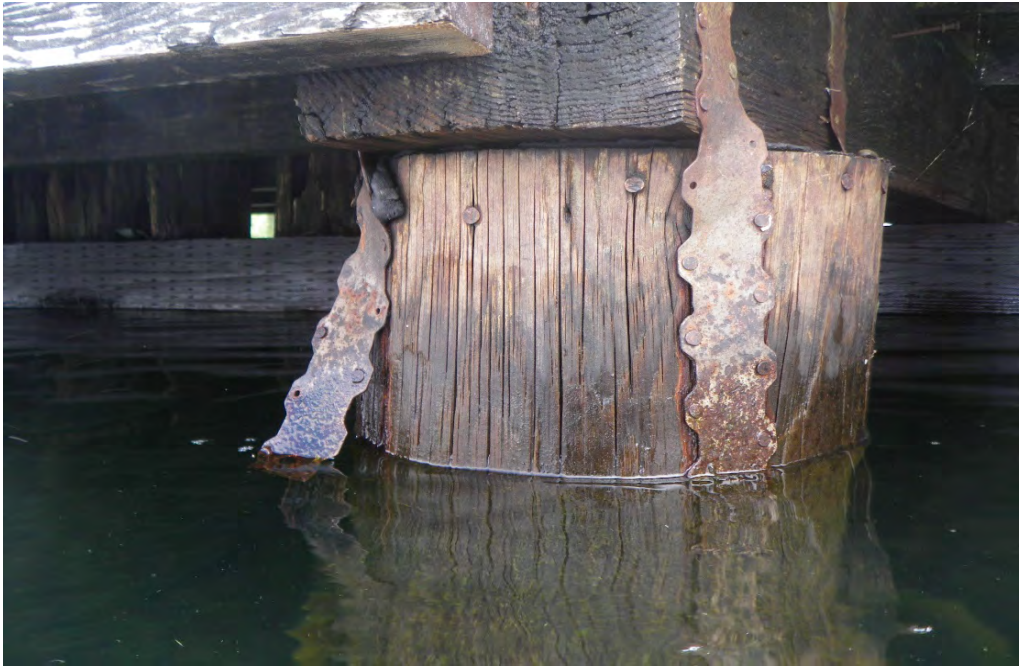
PHOTO No. 7: Bent 36, Row A Pile - Note the moderate to heavy corrosion of the Simpson ties used to secure the pile top / cap connection. Also note that the nails securing the straps are failing and the left strap is not secured. Inspection found the majority of the piles to be treated and to have sustained a minor amount of biological degradation or softening of the outer surface.
