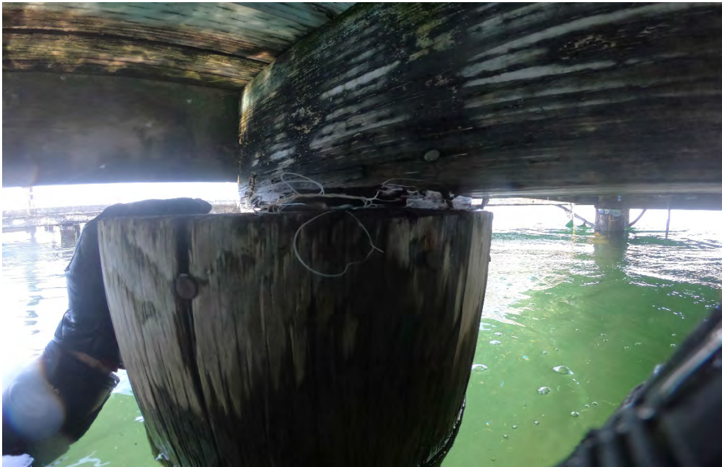
PHOTO No. 5: Bent 15, Row B Pile - Note partial bearing condition of the pile beneath the cap. Inspection noted that the protective metal cover on this pile is missing and the bearing has been estimated at 10%.
