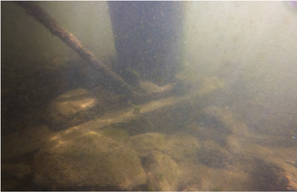
PHOTO No. 9: Bent 24, Row A Pile - Note the large dimension horizontal timbers at the mudline which appear to span between the piles. Also note the steel bracket at the base of the pile and the diagonal tension rod which extends up and is embedded in the poured in place concrete between the two cap timbers.
