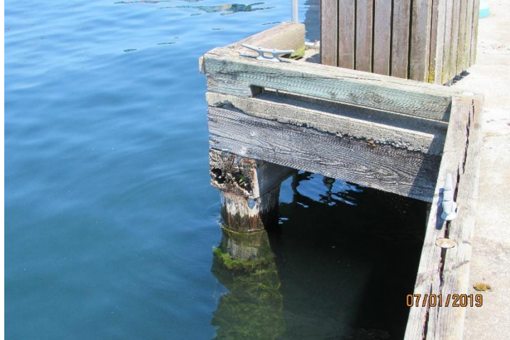
Photo 46. Deteriorated Pile Cap and Bull Rail on Pier (1), 2 nd Ave. South Dock.
