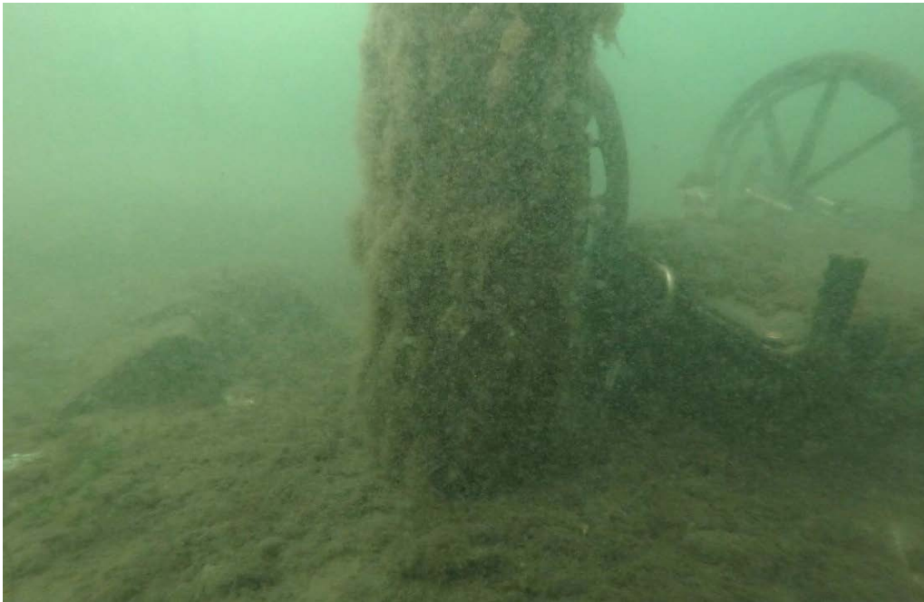
PHOTO No. 7: Bent 16, Row A Pile - Note moderate accumulation of algae on the pile, and the mudline. Also note the wheelchair which has been dumped off the pier. Investigation of the bottom found the bottom to be composed primarily of soft mud and silt at this location.
