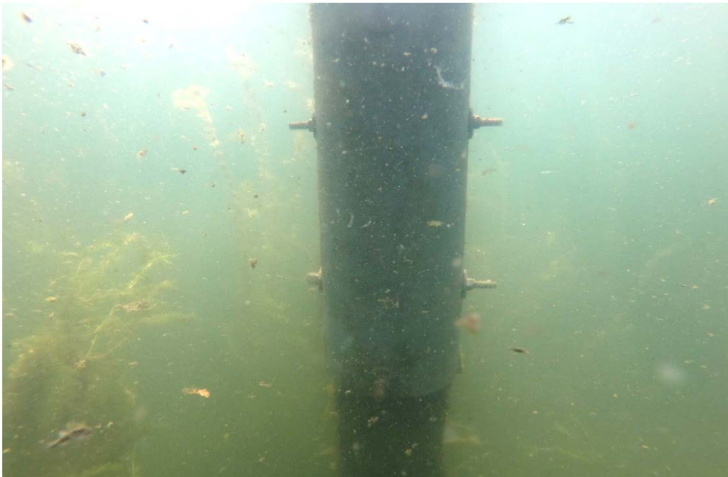
PHOTO No. 15: Bent 51, Row D, Pile Post - Note the overall good condition of the steel sleeve and connection hardware used to secure the splice connection. Inspection of the steel found it to have sustained light to moderate surface corrosion and to be tight.
