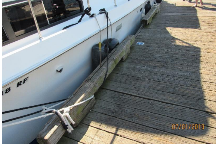
Photo 71. Deteriorated and Damaged Bull Rails and Decking on Pier (8), Marina Park.
