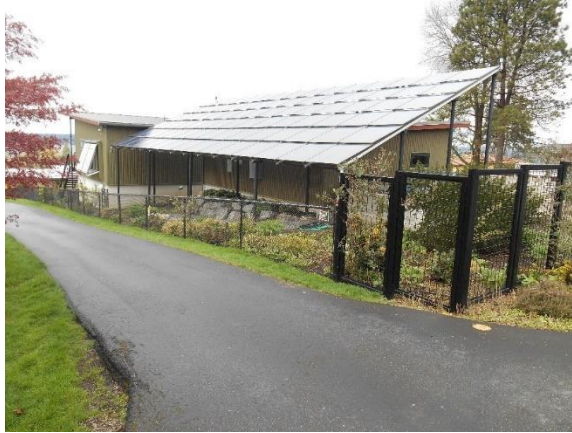
Solar Panel Array
