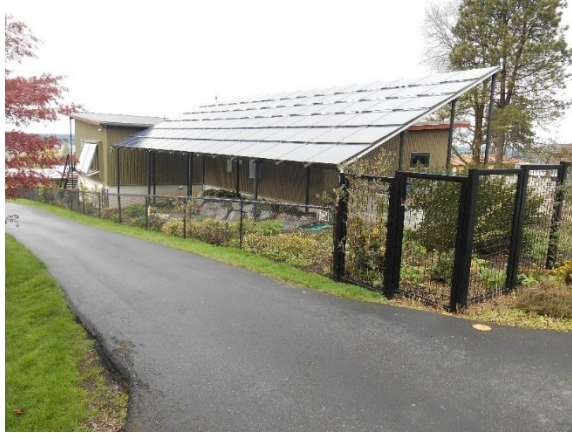
Solar Panel Array
