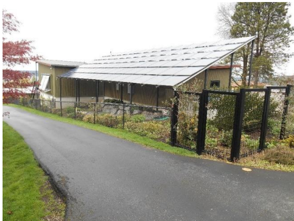
Solar Panel Array
