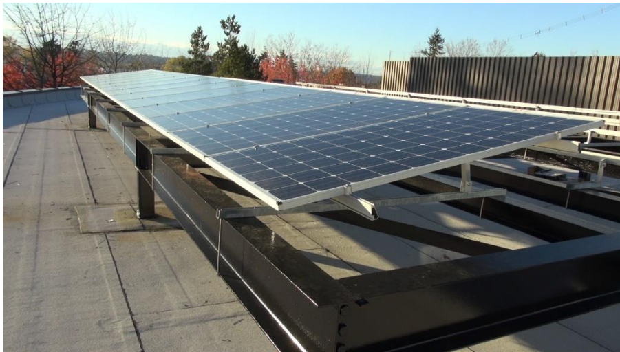
Solar panels on the roof of City Hall
