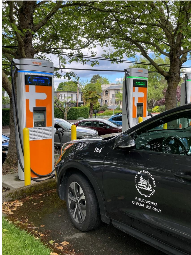
Electric Vehicle charging stations at City Hall
