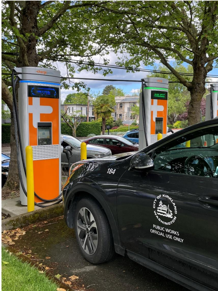
Electric Vehicle charging stations at City Hall
