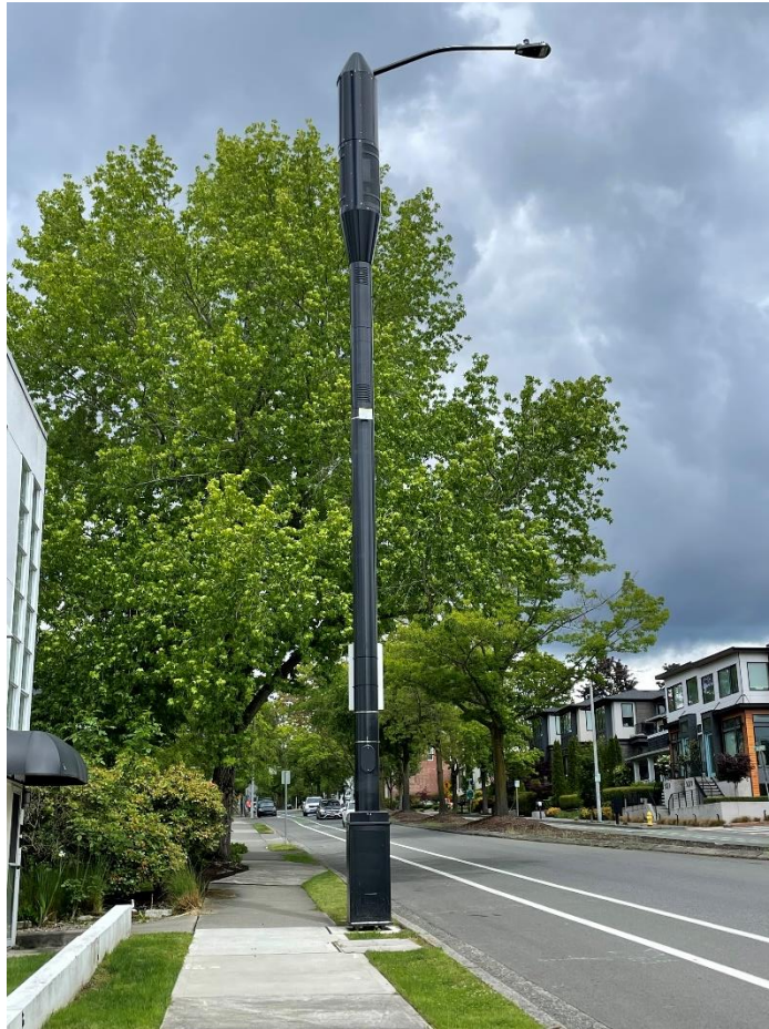
Wireless service facility shrouded within a light pole
