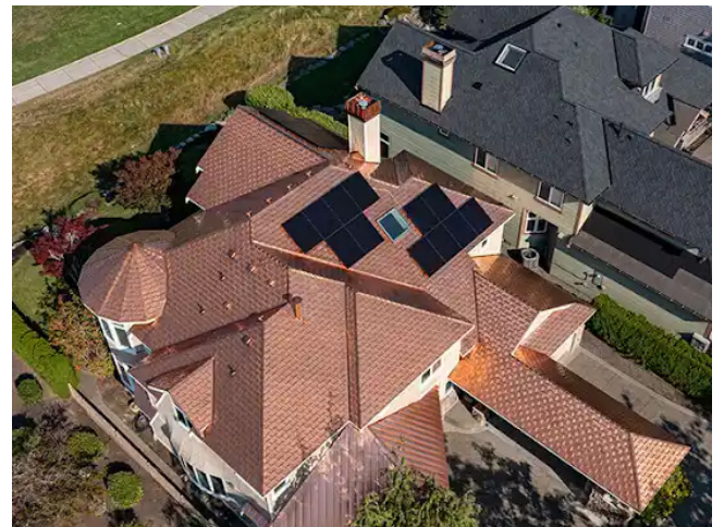
Residential Solar Panels
