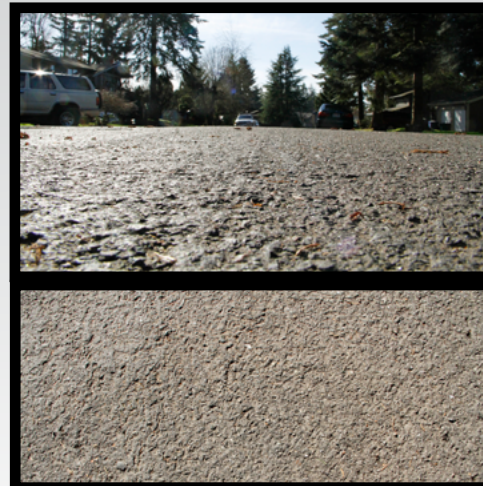
Street: 91 st Court Northeast Sealed: Aug. 30, 2016 Photo: April 3, 2017
