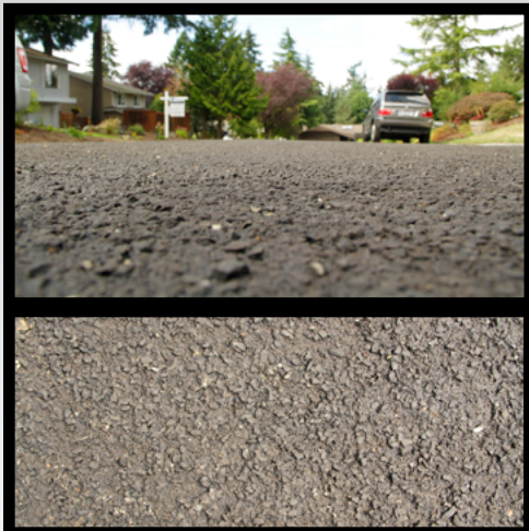
Street: 91 st Court Northeast Sealed: Aug. 30, 2016 Photo: Sept. 8, 2016
