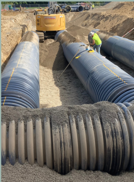
Above: Storm detention at Rose Hill Elementary School.
